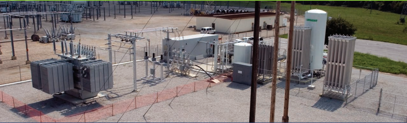
AEP's Bixby substation in Groveport, Ohio
